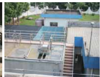
Facilities for treating sewage water (DMGZ)
