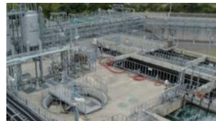
Wastewater treatment facility (Zenmyo Plant)
