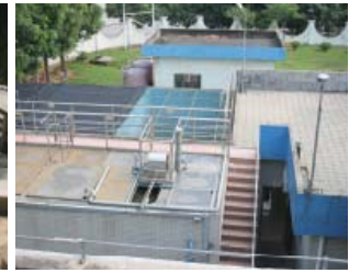
Facilities for treating sewage water (DMGZ)
