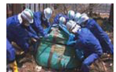
Associates carrying out recovery work at disaster-affected areas of the Great East Japan Earthquake
