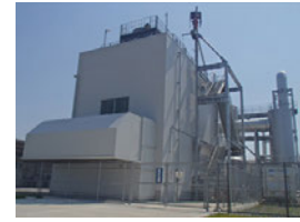
Co-generation facilities at the Nishio Plant (south facility)
