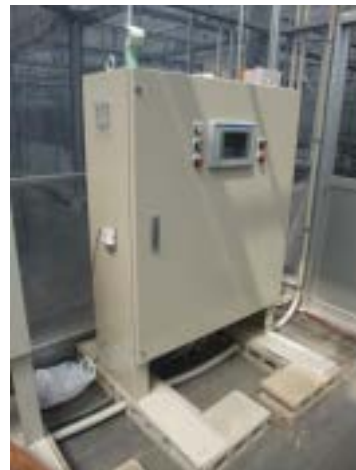
Environmental control system
